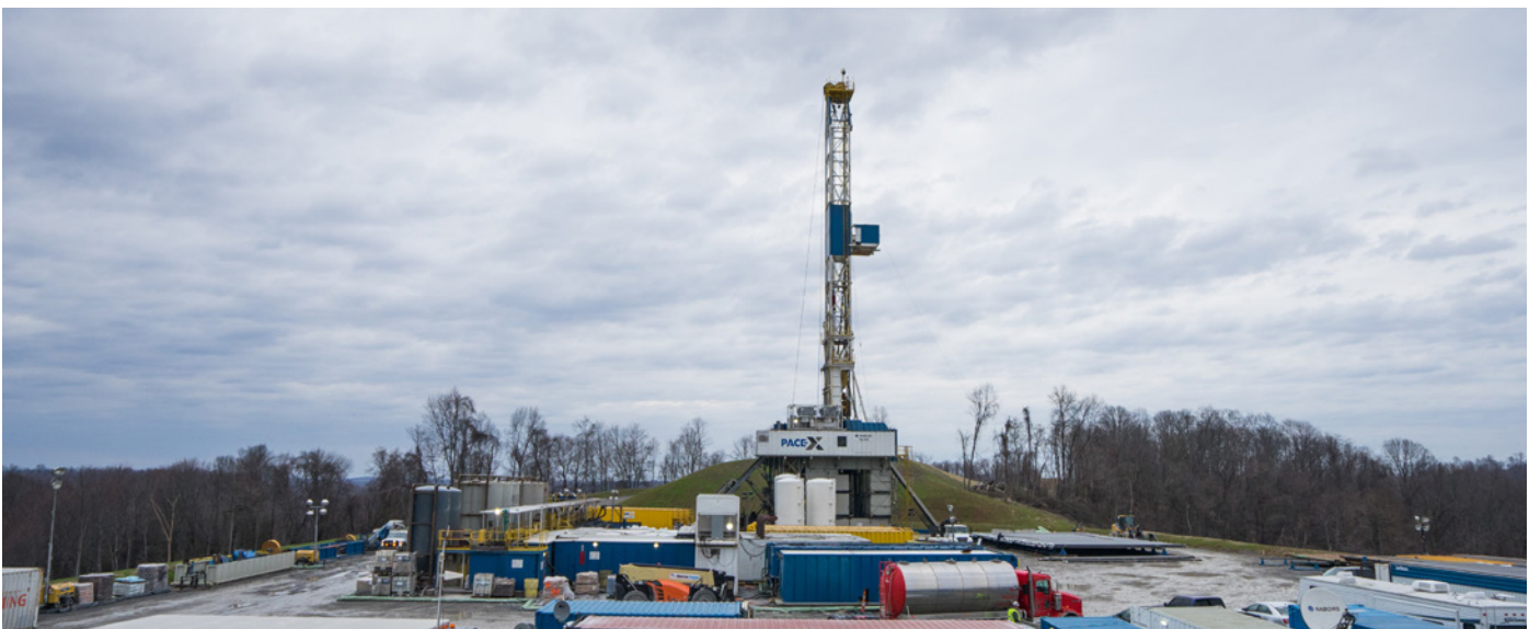
A view of the Marcellus Shale Energy and Environment Laboratory – a dedicated FE field laboratory at the Northeast Natural Energy production site in Morgantown, West Virginia. The project provides a resource to develop and validate new knowledge and technology to improve recovery efficiency and minimize environmental impacts of unconventional resource development.
